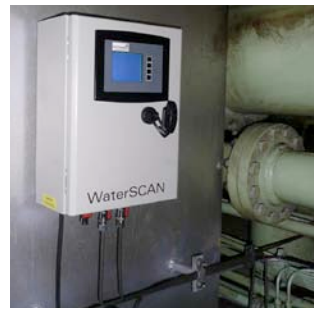
A typical marine installation
